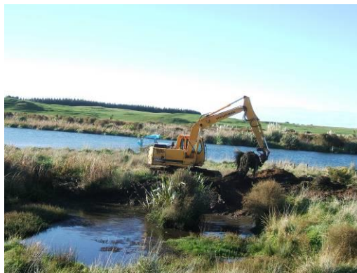
Photo 4. Enlarging the end of the feeder channel to make the east new pond.
